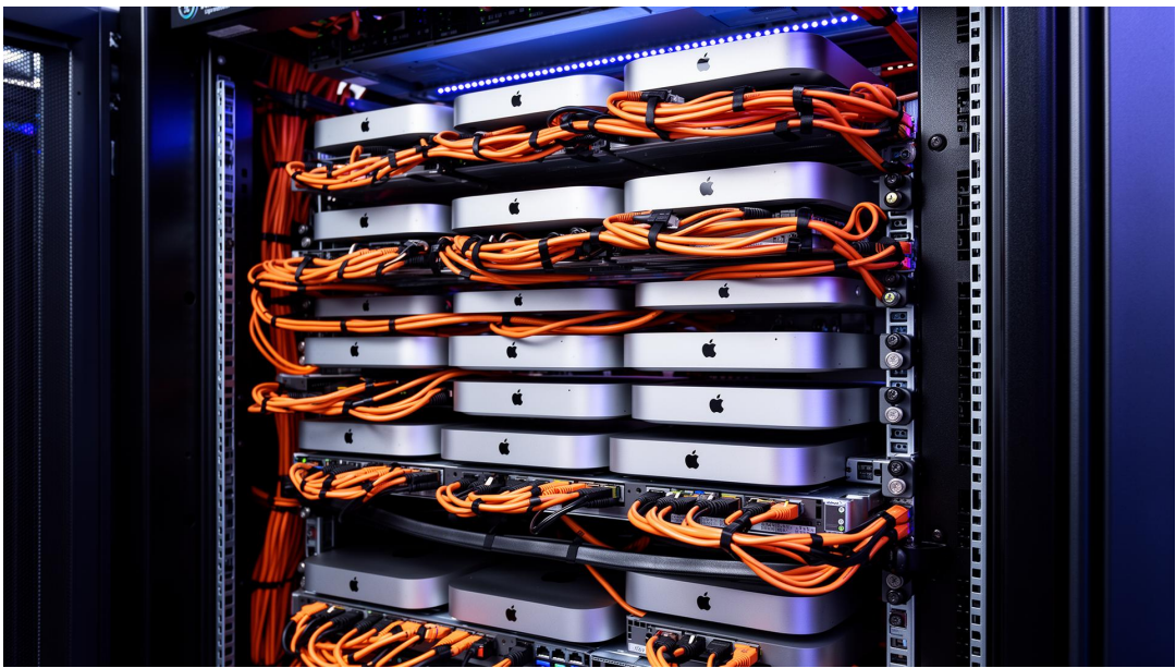
Custom 1U trays, colour-coded cabling and dual-feed PDUs in our private cages.
